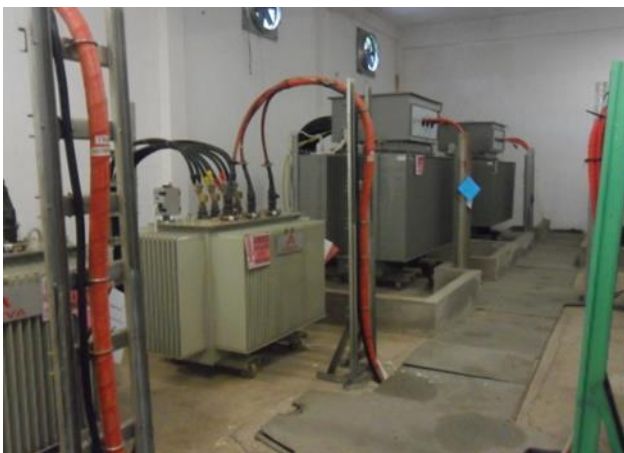
Gambar 4. Transformator TM (main power house)
