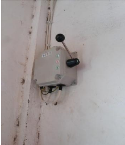
Gambar 4. Manual Transfer Switch
