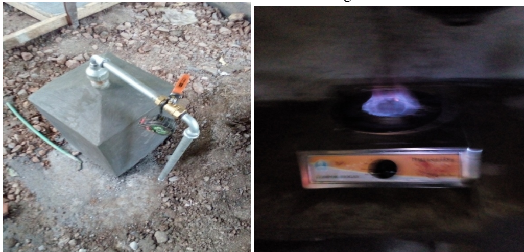
Gambar 3 . Instalasi Bio gas
