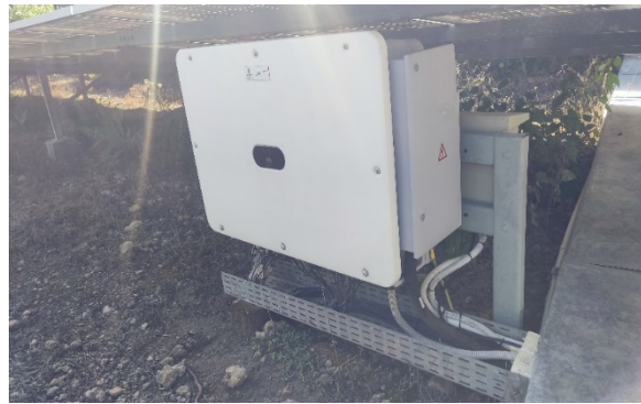
Gambar 4. Inverter Huawei Sun2000-100KTL
