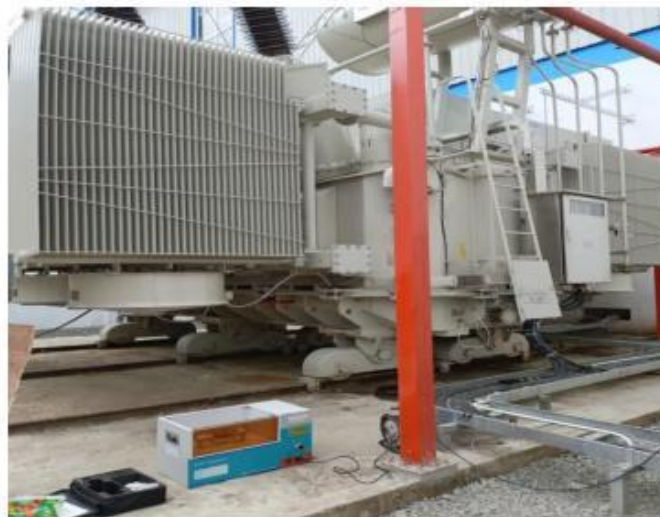
Gambar 1. Power House PLTA MALEA 2x45 MW
