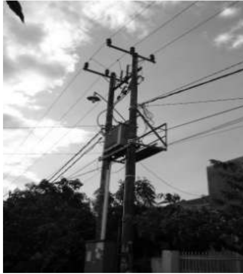
Gambar 2. Jaringan trafo distribusi TR 220V/380V/100KVA
