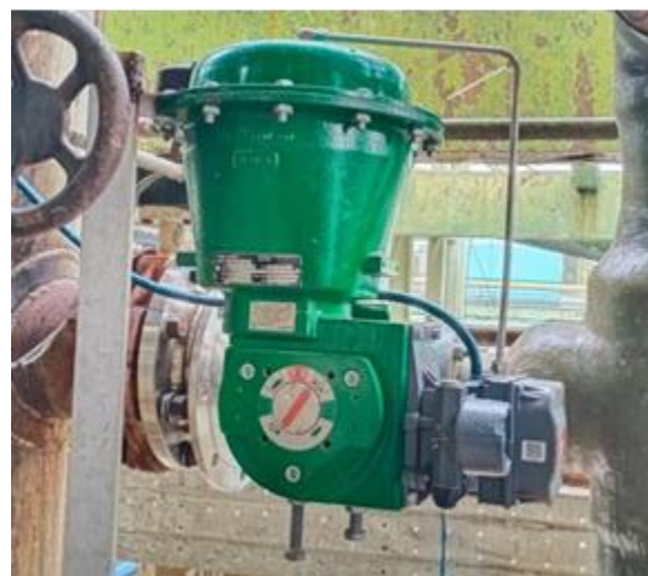
Gambar 6. Opening control valve
