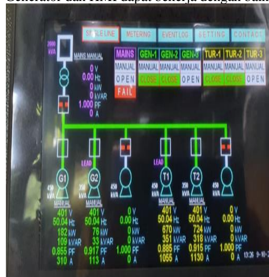
Gambar .9. Hasil Panel HMI Power Meter
