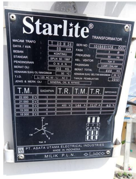
Gambar 5. Name Plate Trafo Distribusi GD 651BB
