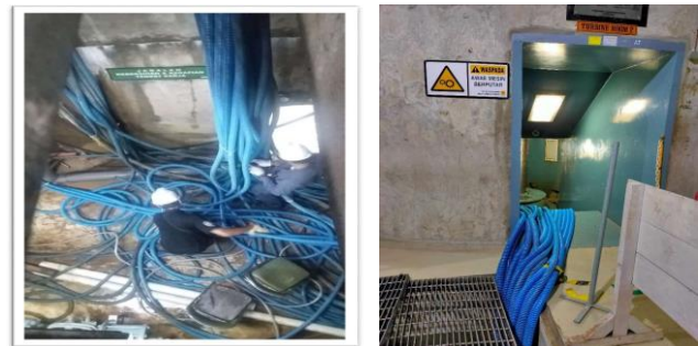
Figure 1. Leakage conditions in the turbine pit
